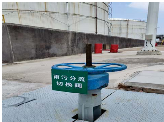
储罐区雨水分流切换阀
